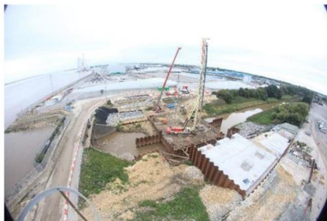
Two pumps in operation October 2023, East Hull pumping station
